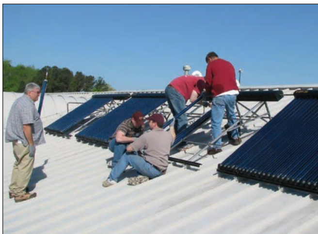
People are the solution. ASHRAE volunteers involved in the Community Sustainability Project program at work in their local community.
